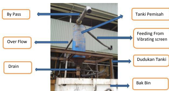
Gambar 9. Oil Trap Tank
